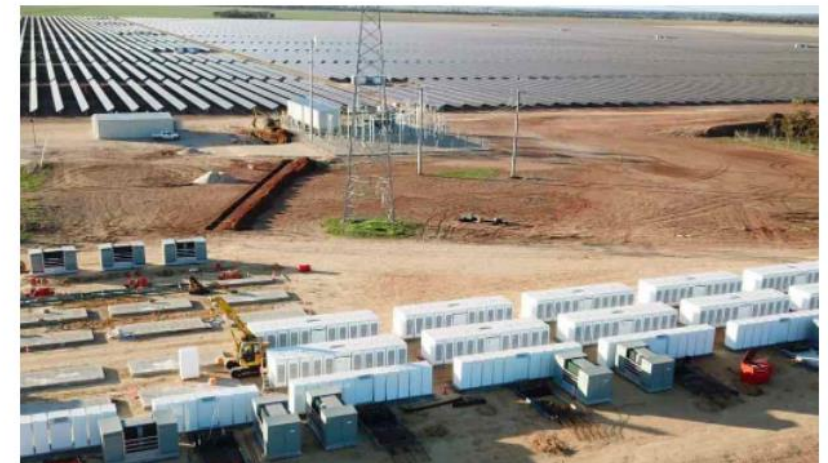
Gannawarra solar farm and battery storage facility. Source: Wirsol
