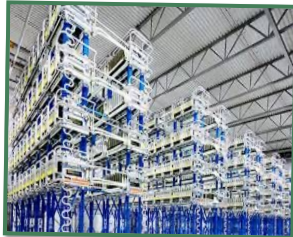
HVdc Substation (2,400 PE modules, 100 – 3,000 MW)
