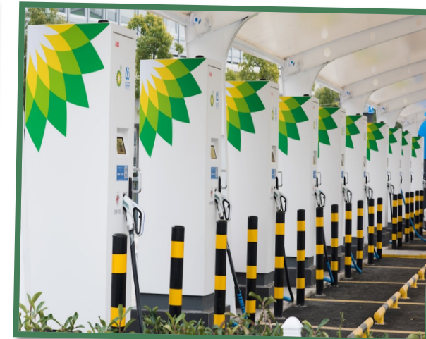
EV Charging Stations (300 chargers in T&D grid)
